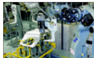
Figure 2—Mazda's new friction stir welder making a weld on a body assembly.
