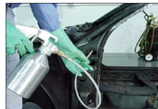
Figure 1—Epoxy primer is being applied inside of this A-pillar to ensure corrosion protection.
